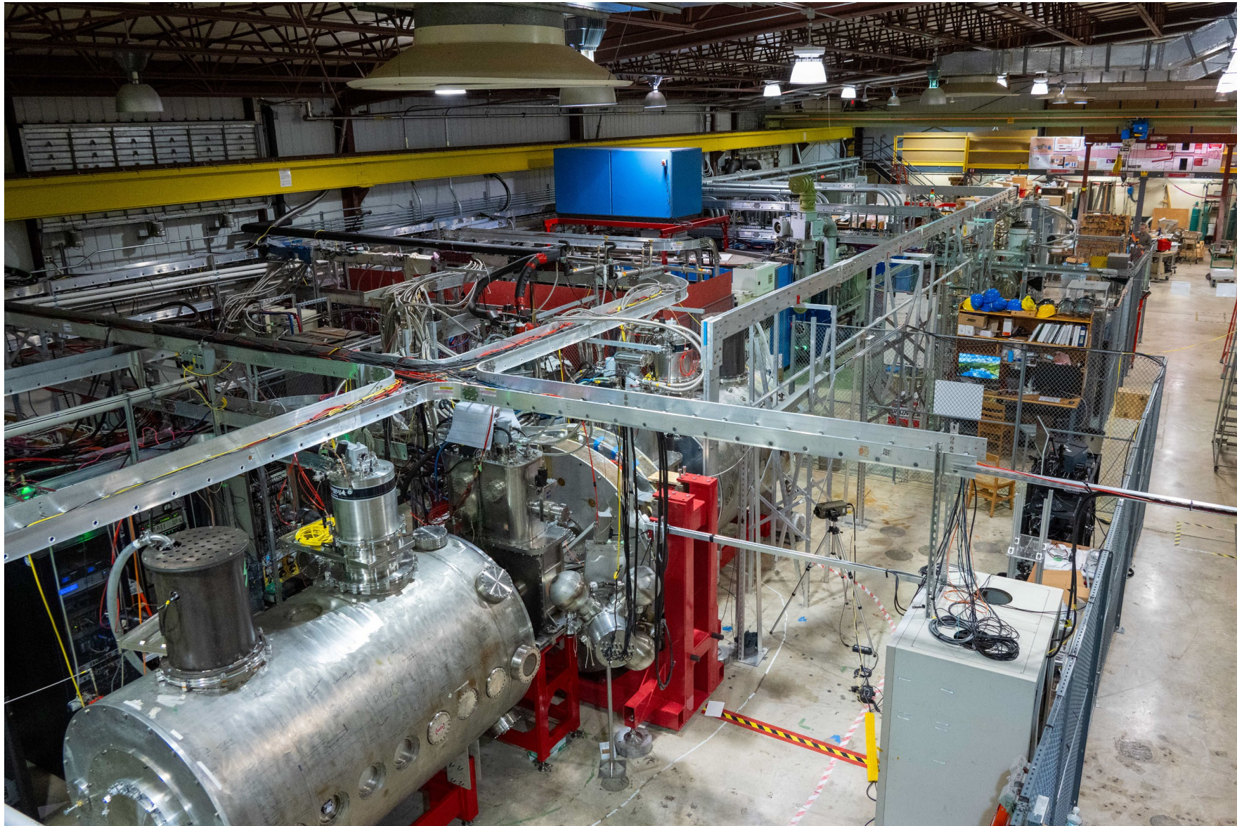
UW-Madison, KRC-SRC Rowe WHAM Plasma Physics Lab Electrical and Cooling Upgrade Project budget: $3.2M. Substantial Completion: November 2024
