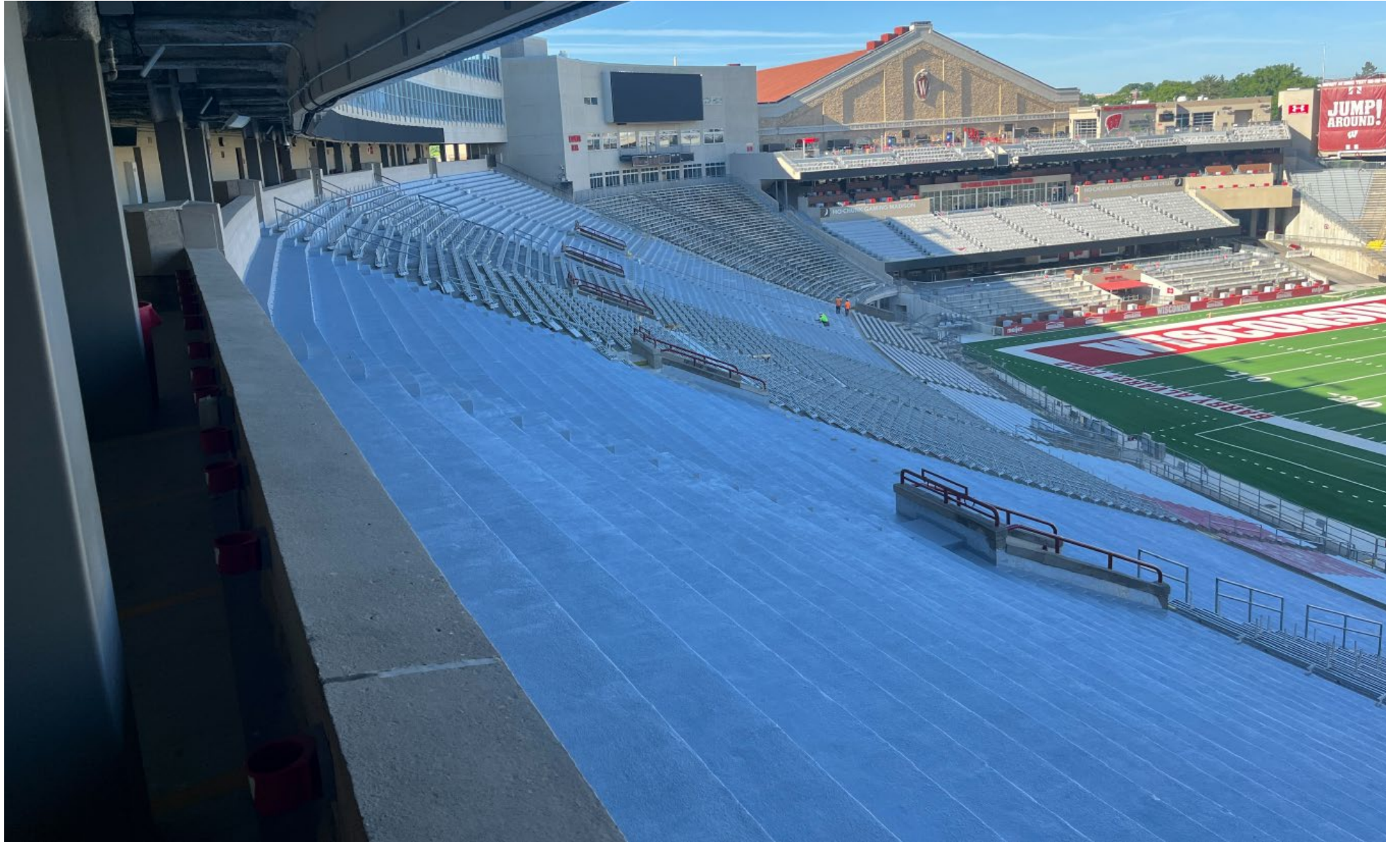
UW-Madison, Camp Randall Stadium East Bowl Recoating Project budget: $2.4M. Substantial Completion: May 2025
