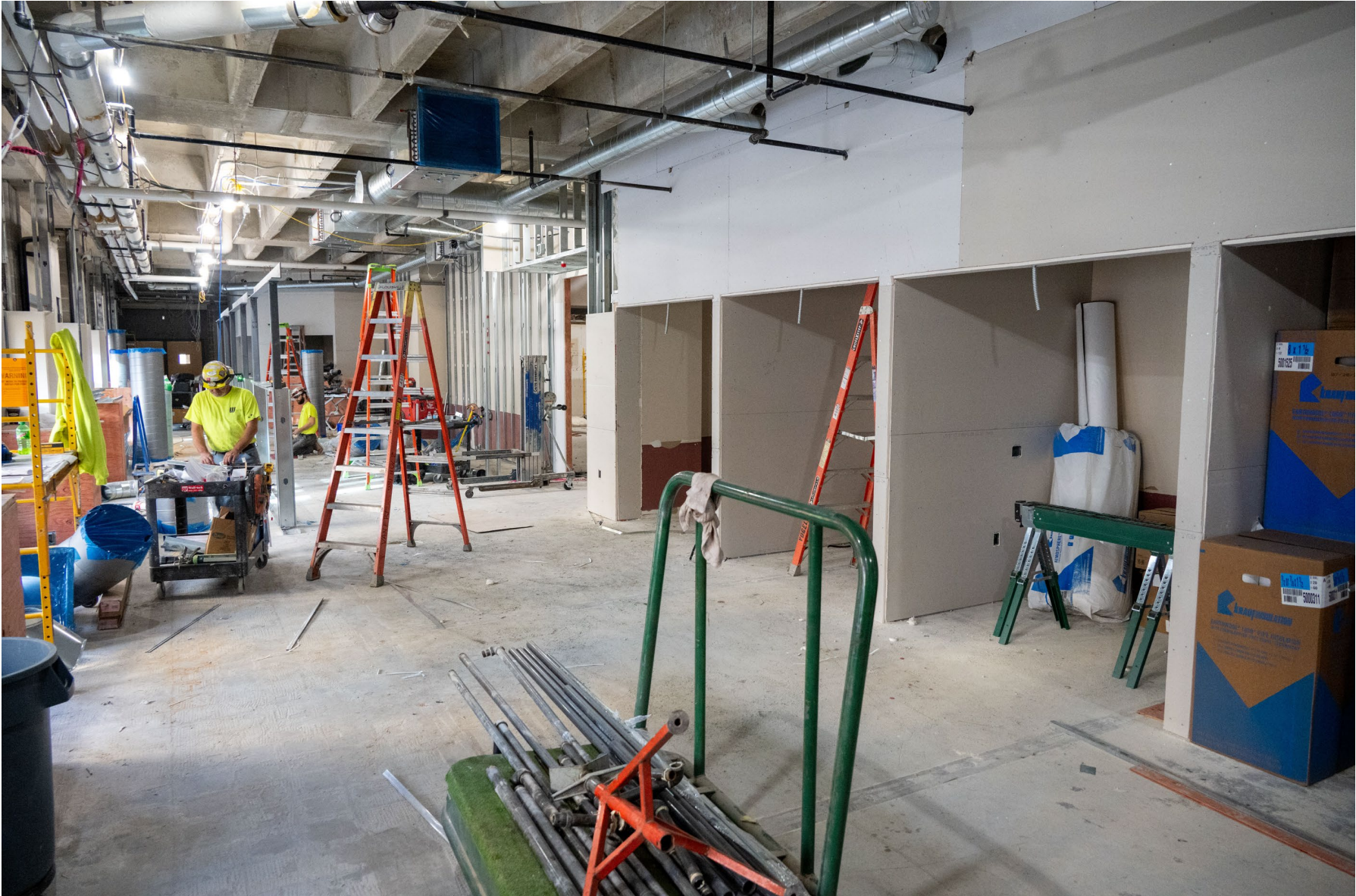
UW-Madison, Grainger Hall 2nd and 5th Floor Renovation Project budget: $8.8M. Substantial Completion: March 2025
