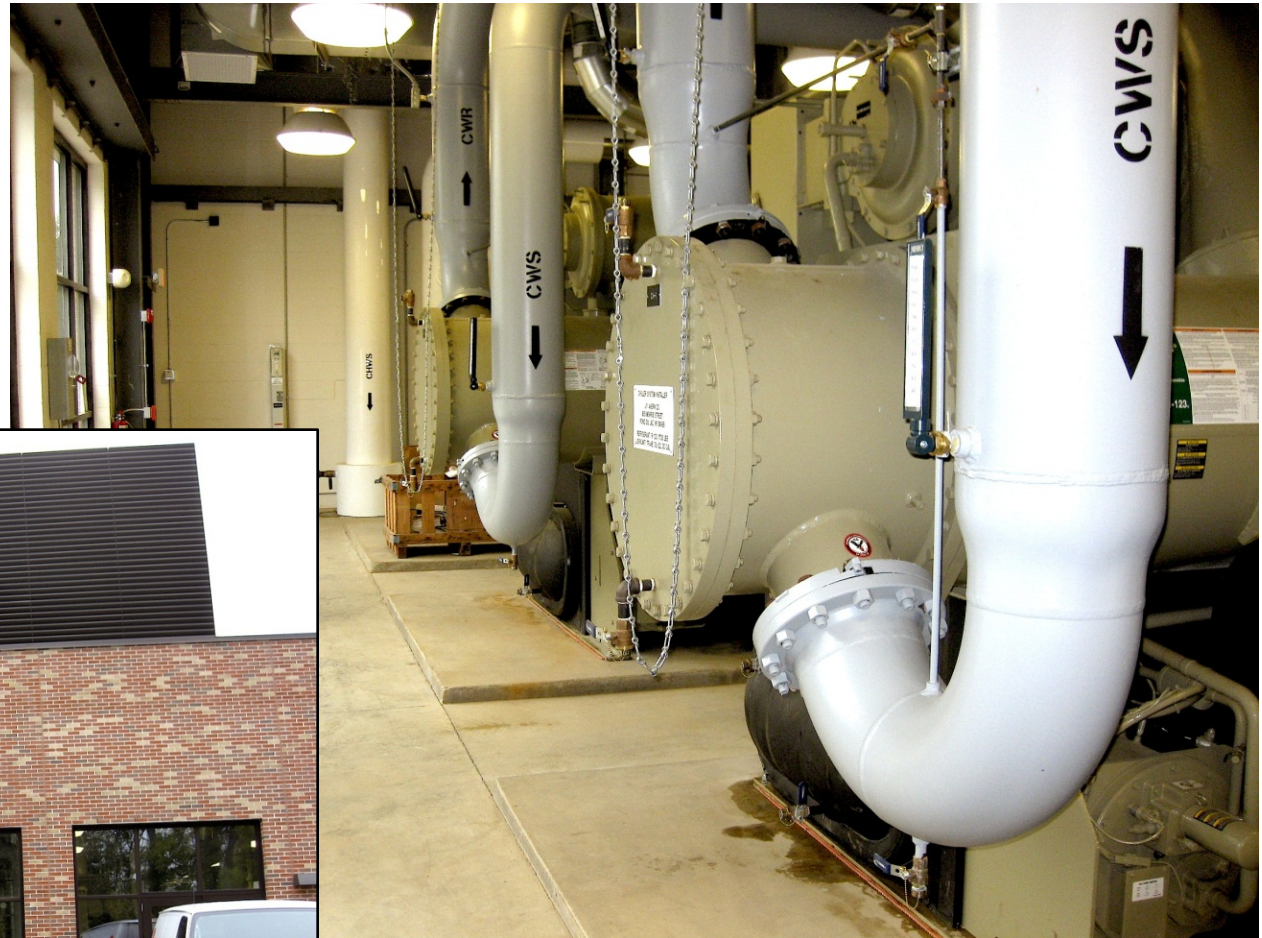
Chilling Plant - Interior
