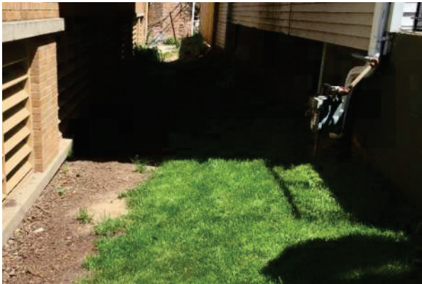
Photo 1. Drain from adjacent building discharges out on grade
