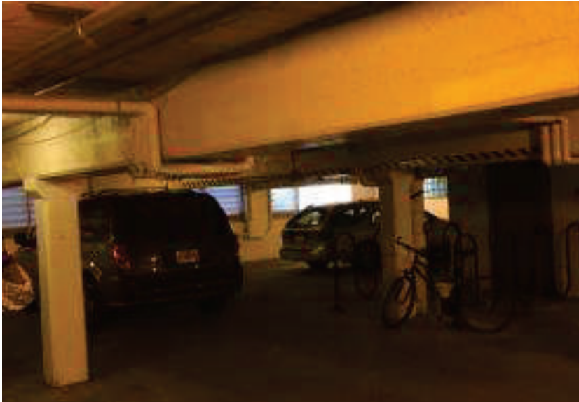
Photo 6. Low ceiling clearance in the garage. Exposed pipes freeze during winter
