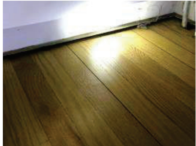
Photo 9. Settlement at west elevation on 3 rd floor
