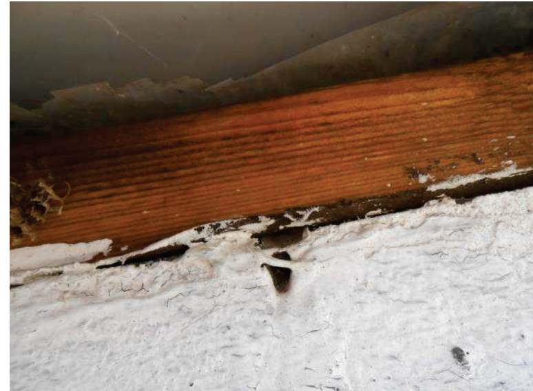
Photo 22. Example of wood blocking under metal coping
