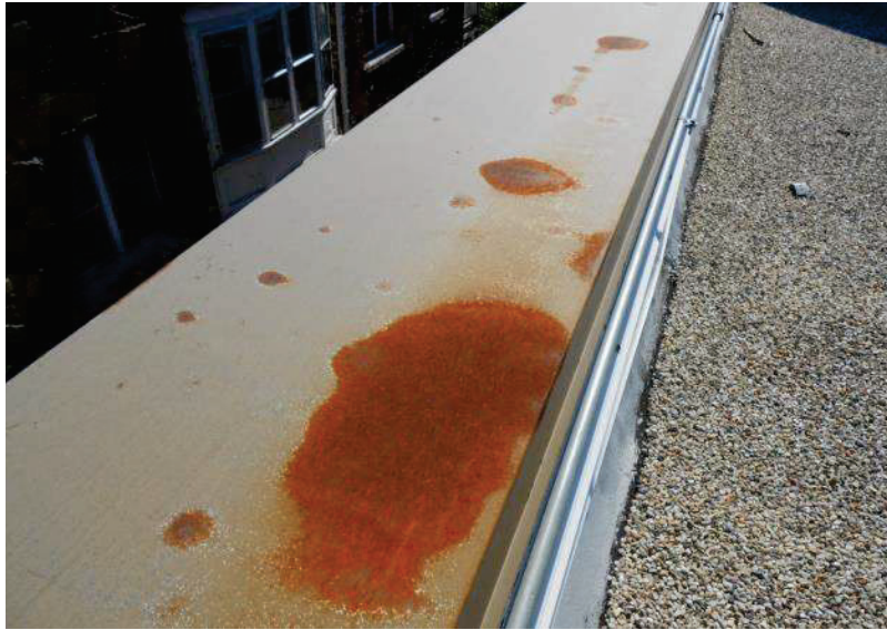
Photo 21. Example of corrosion on metal coping
